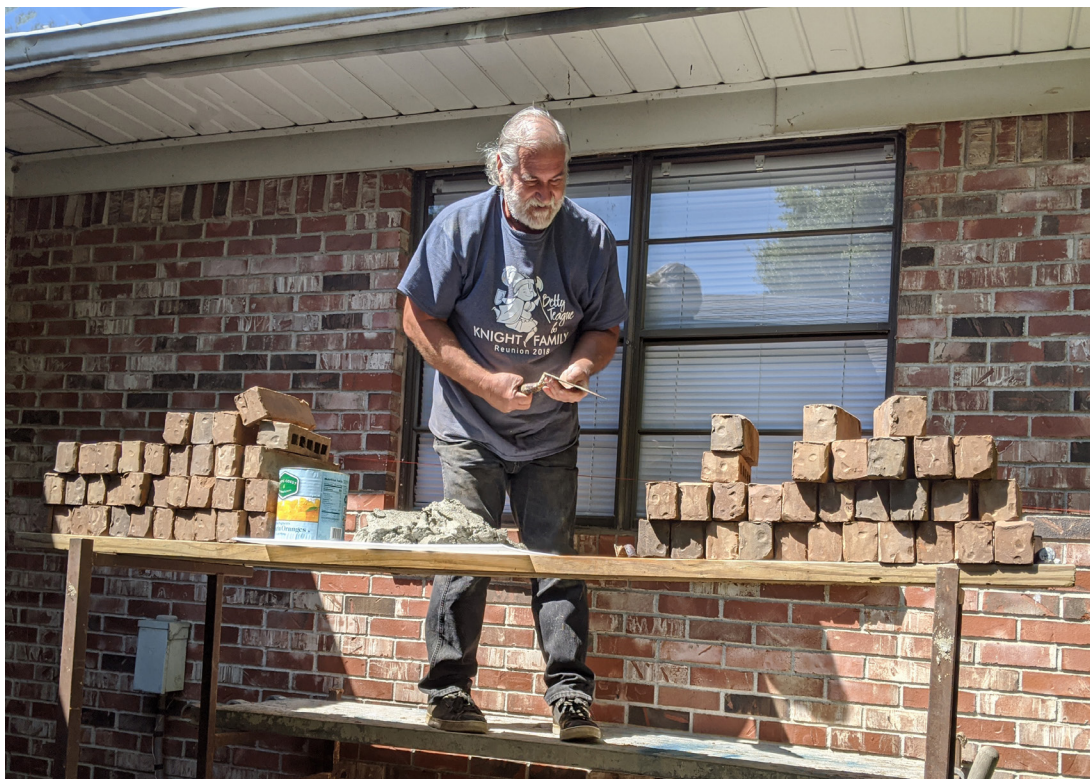
Volunteer Terry Whitaker bricks in a window for security and light eradication at the building (formerly a duplex) where our new digital assets department will be located.
