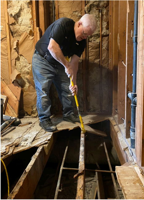
Facilities manager Walt Gallagher removes old flooring to make way for plumbing repairs.
